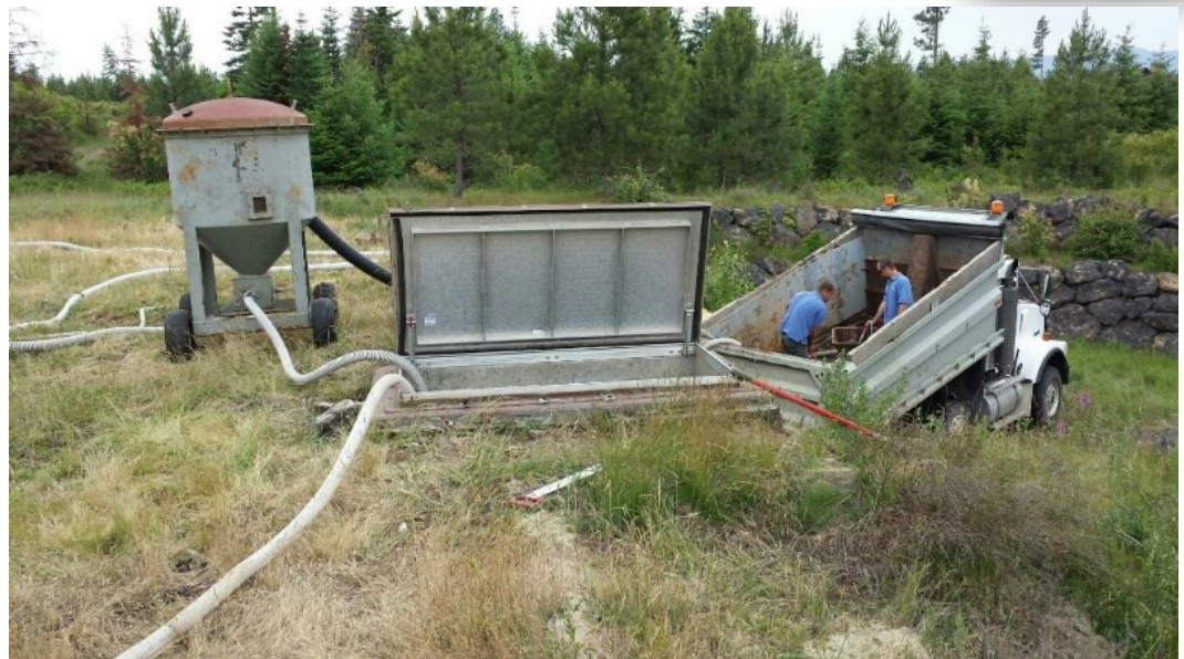
Two of North Kootenai Water District's Service Technicians in one step of cleaning sand filter beds at Gozzer Ranch. On the left is Jesse Camburn and to the right is PJ Lockler.
